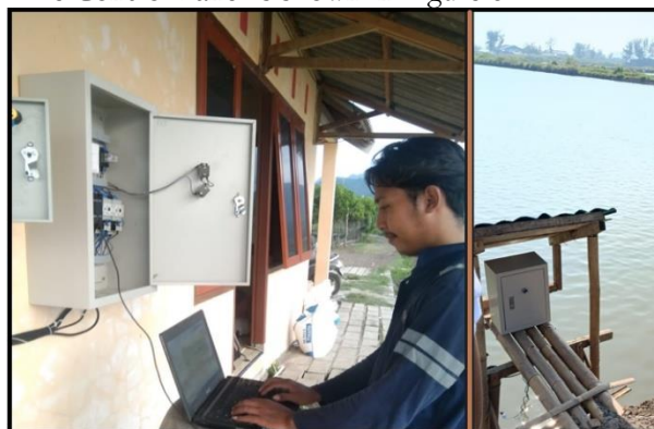
Figure 6. SSDP (Control Panel)
