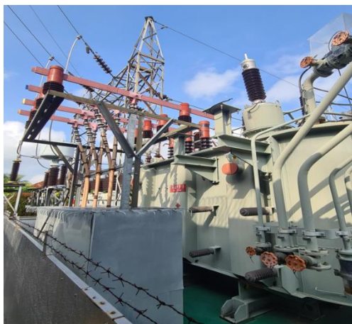
Figure 2. Transformer 1, 30 MVA 70/20 kV at Bungaran Substation, Palembang.
